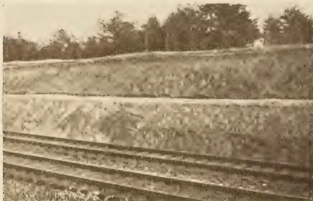
FIGURE 14.—TERRACING OF FACES OF RAILWAY CUT IN CLAY, BETWEEN WASHINGTON AND BALTIMORE. SURFACE DRAINAGE IS PROVIDED FOR ON EACH TERRACE. ONE OF THE METHODS USED TO PREVENT SLIDING IN CUTS
